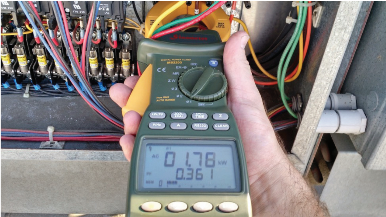
Technical Appendix H: Example photo of the condenser fan spot measurement
